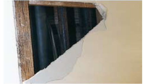
Asbestos insulating board (AIB)
