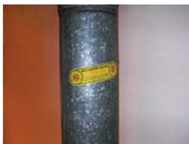
Figure 43 Metal clad gas flue containing chrysotile lining
