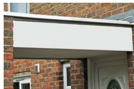
Figure 15 AIB panel in porch
