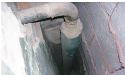
Figure 9 Lagged pipe in wall cavity
