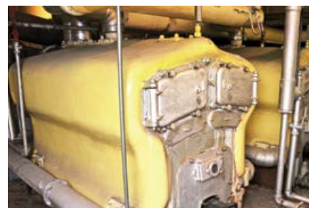
Figure 13 Amosite lagged boiler with hard plastic coating
