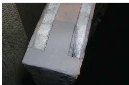
Figure 14 Asbestos panels inside fire door
