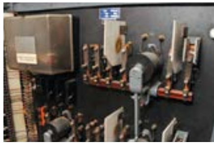
Figure 50 Open electrical switchboard with asbestos flash guards
