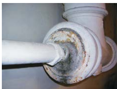
Figure 30 Amosite and chrysotile packing on waste pipes
