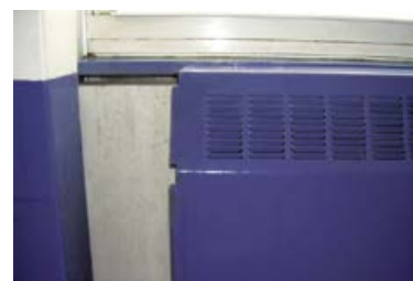
Figure 19 AIB behind school radiator unit
