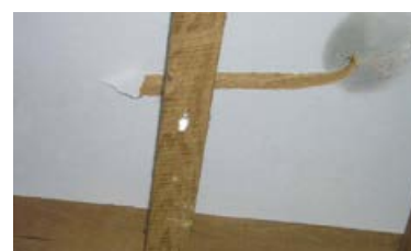
Figure 25 Chrysotile paper on strawboard ceiling panels
