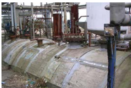
Figure 12 Lagging on large petrochemical vessel
