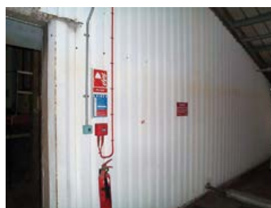
Figure 38 Chrysotile/bitumen coating under metal cladding
