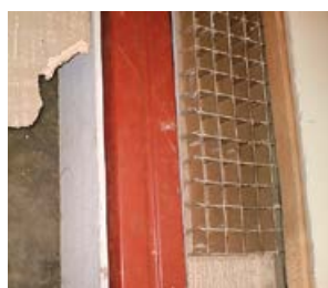
Figure 21 AIB column fire protection in CLASP building
