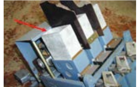
Figure 49 Electrical switchgear with asbestos flash protection
