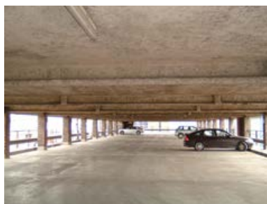
Figure 7 Sprayed limpet on car park roof
