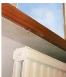
Figure 20 AIB panel between radiator and window
